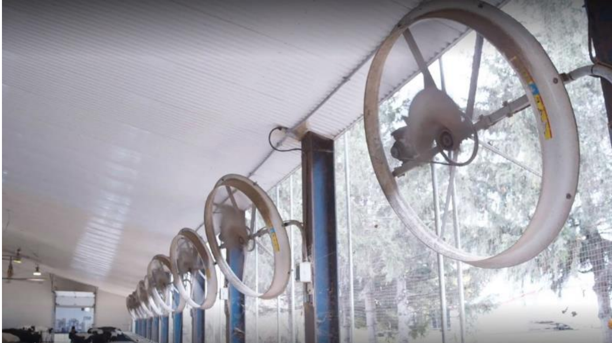
Figure 6. LVHS fans placed along the side of the building pulling air into the barn through the sidewall air inlets, Source: Ferme Caribou.
