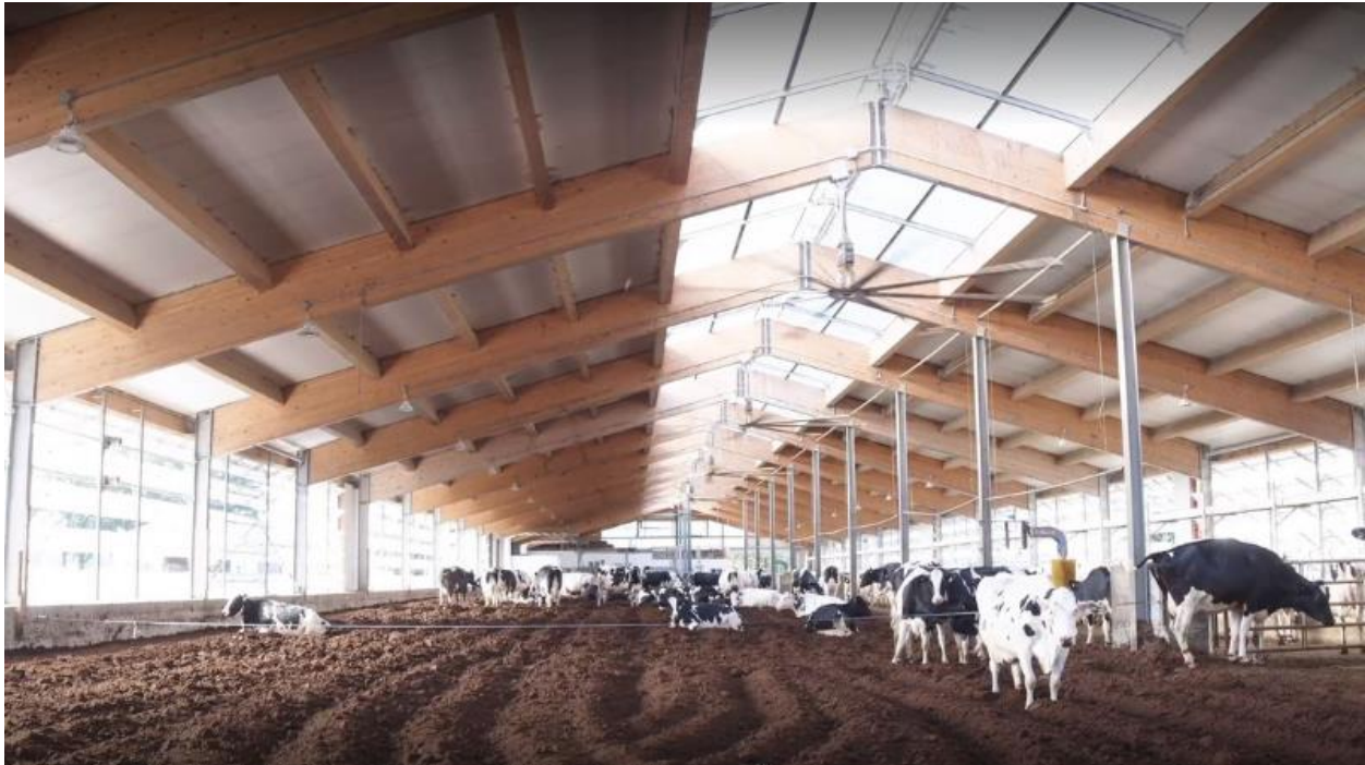
Figure 2. Naturally ventilated barn with added HVLS fans to increase air speed under the fans to assist in cooling dairy cows, Source: Craven Farm.
