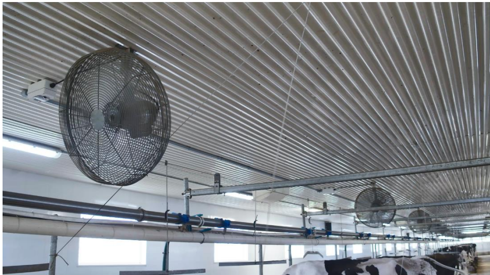
Figure 12: Addition of circulators above tie-stalls to ensure proper air speeds reach the cows in their stalls, Source: Ferme J.C. Lafortune et fils inc.
