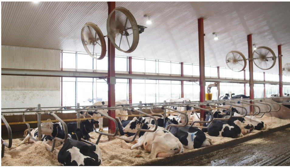
Figure 7. LVHS recirculation fans positioned above the cows' stalls (resting area), Source: Ferme Melga Inc.
